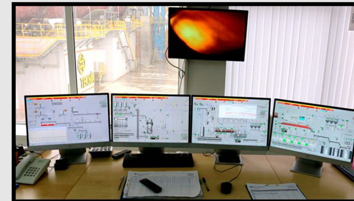
CCR - Central Control Room
